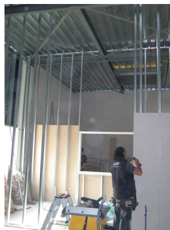
Photos: left: overview of the building, the lighter grey part shows the location of the microscopes. Right: construction worker makes a wall for the microscope control room.
