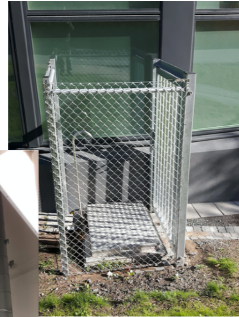
outside: exhaust for N gas
